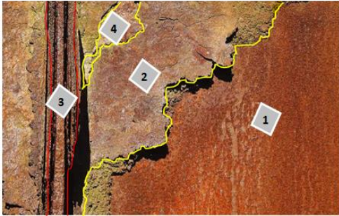
Fig. 13. Types of corrosion in the structure of the lighthouse: 1- Uniform corrosion, 2- irregular Corrosion, 3- Galvanic Corrosion, and 4- Stress Corrosion Cracking (SCC).
