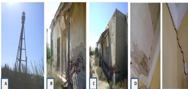
Fig. 14. Many forms of deterioration Researcher 2023
