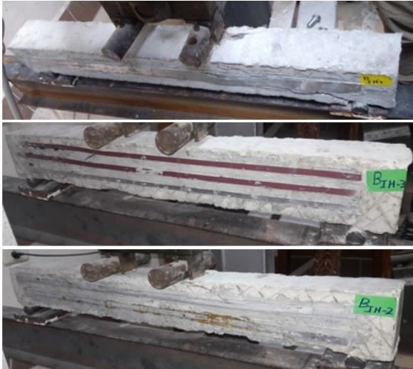
Fig. 13. Crack pattern and mode of failure for the beams strengthen using strengthening technique (4).
